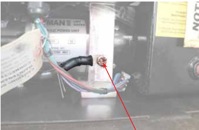
Ground to Side of Power Unit
